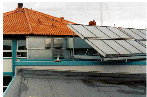
Figure 2: Solar assisted desiccant cooling system Riesa: collector and air handling unit installed on the roof
