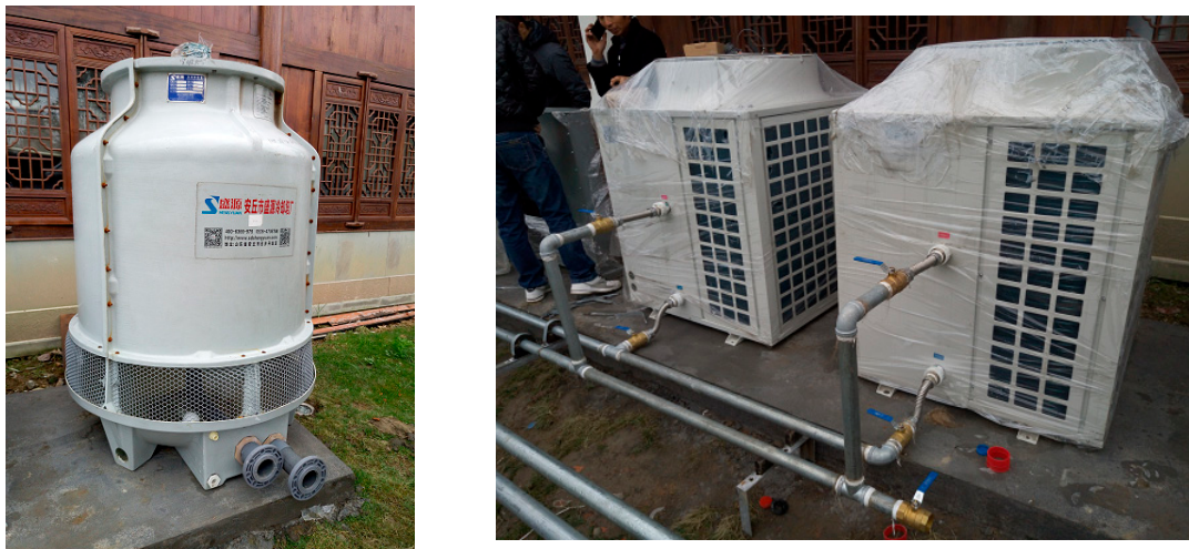
Figure 6. Photos of the (left) cooling tower and the (right) two heat pumps.
