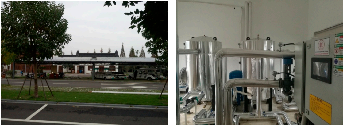
Figure 5. Photos of the (left) solar collector field on the roof of a steel-structure parking shed and the (right) equipment room.
