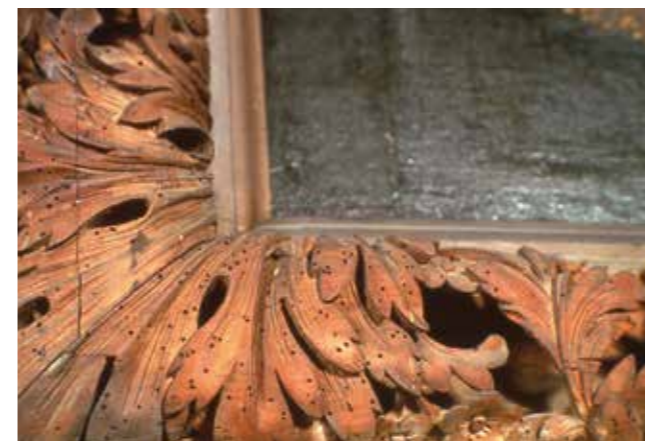
Woodworm damage (National Trust Images)
