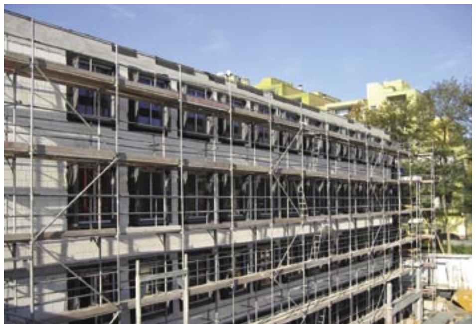
Straight lines: Numerous windows in the exposed concrete facade of the new institute building (currently still hidden by scaffolding) will make for well-lit, friendly offices.
