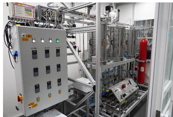
Fig. 3: Hydrogenation plant technical center
