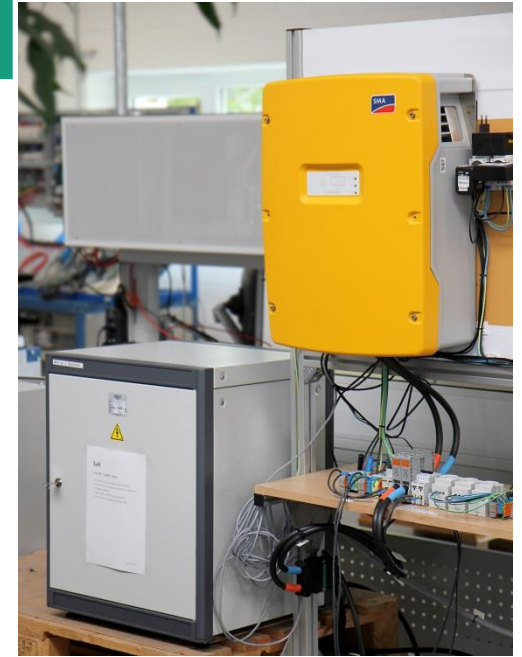
SMA components with SAFT Battery
