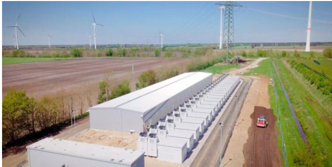
Abb. 11 Batteriespeicher Jarjelund (pv magazine, 2022)
