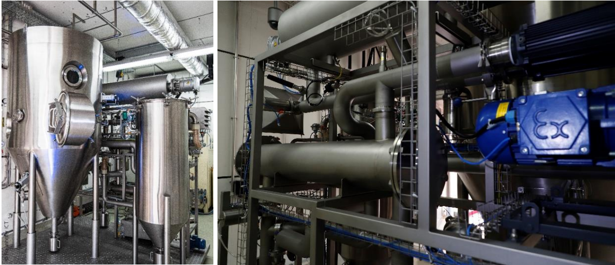
Figure 3: Spray tower (left) and solvent recovery system (right)
